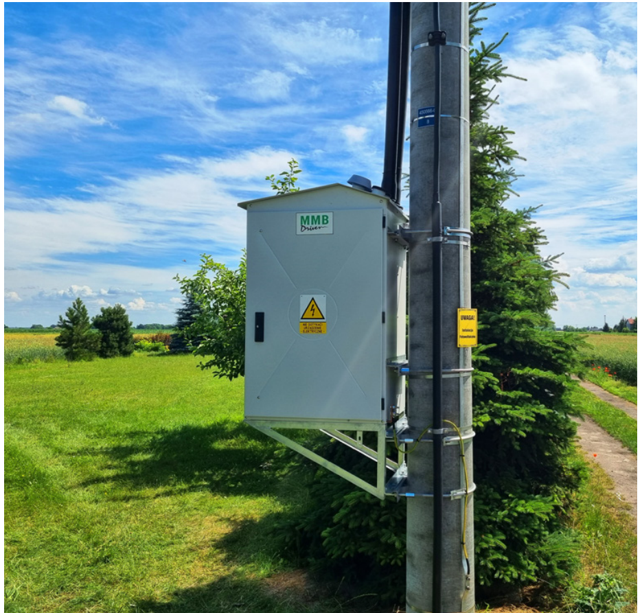
Pic. MMB SmartGridEnabler installed on a pole
